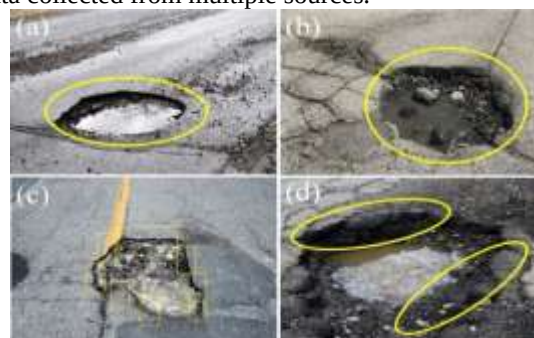
Figure 3. CNN edge detection system to identify the pothole on the road surface
