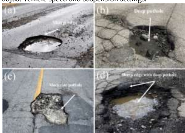
Figure 1. Different types of potholes on the road surface
